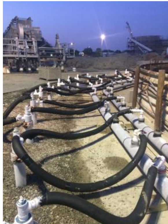
Figure 8. Refrigeration Pipe System
