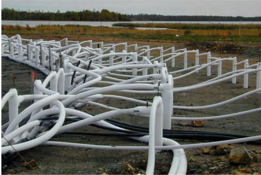
Figure 14. Noranda Crown Pillar Excavation Project, Quebec, Canada - three rows of freeze pipes
